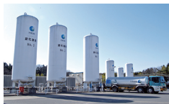
On-site bulk supply
