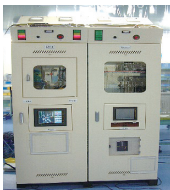
Gas dilution supply facility
