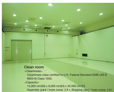
Inside clean room
